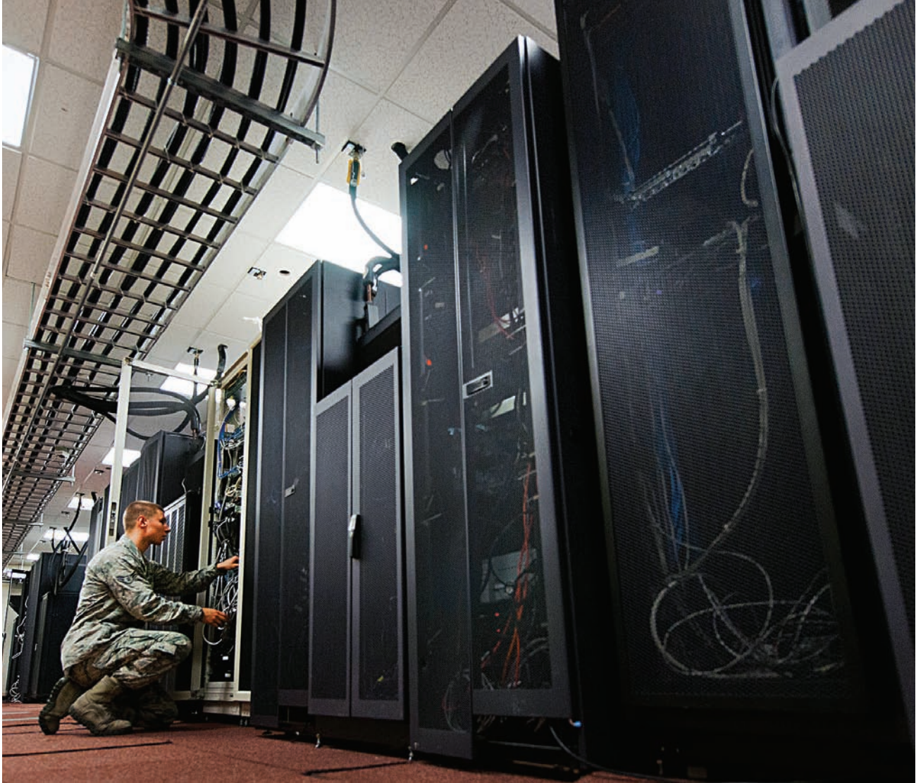
Airman 1st Class Nick Fazio verifies the status and configuration of the 96th Communications Squadron's data center equipment at Eglin Air Force Base, Florida. Approximately 40 airmen and civilians are responsible for the connectivity of the base's more than 19,500 user workcenters. DARPA spintronics research enabled transformative technologies that have become the backbone of data storage today.
