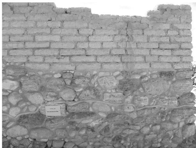
Fig. 4: Mudbrick walls with fieldstone foundations and lower wall. Photo by Ian Scott, creative commoms.
